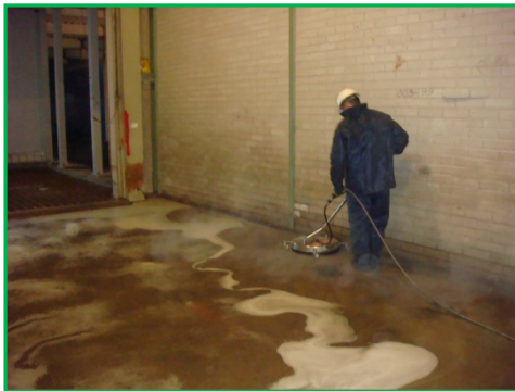
Pic. 15: Using the floor spinner to get the hot detergent / water mix with high pressure (100°C; 300bar) into the concrete to ensure removal of the oil to a sufficient depth (2-3cm)
